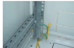
Bottom part of the rack—detail
